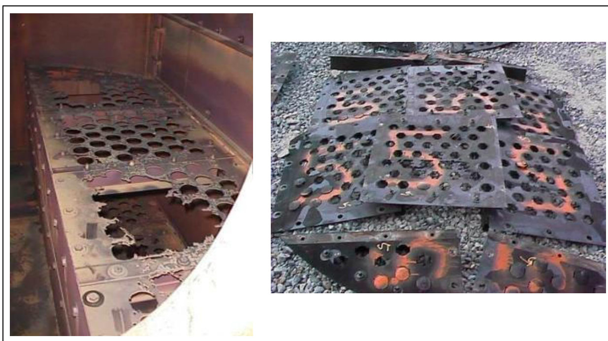
Figure 2: Examples of uniform corrosion on AISI 410 internals in sweet service amine unit [4].
